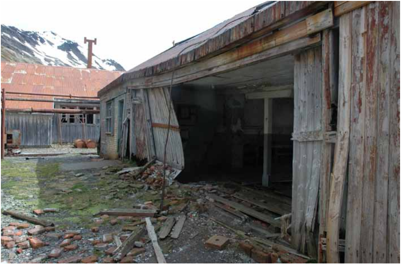
14.4 The collapsing west end of the south wall
