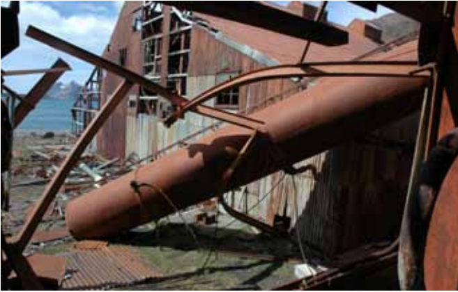
5.2.4 Collapsed boiler chimney seen from the Boiler House
