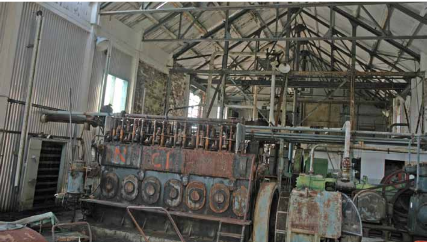
5.2.7 Diesel generators in the Power House
