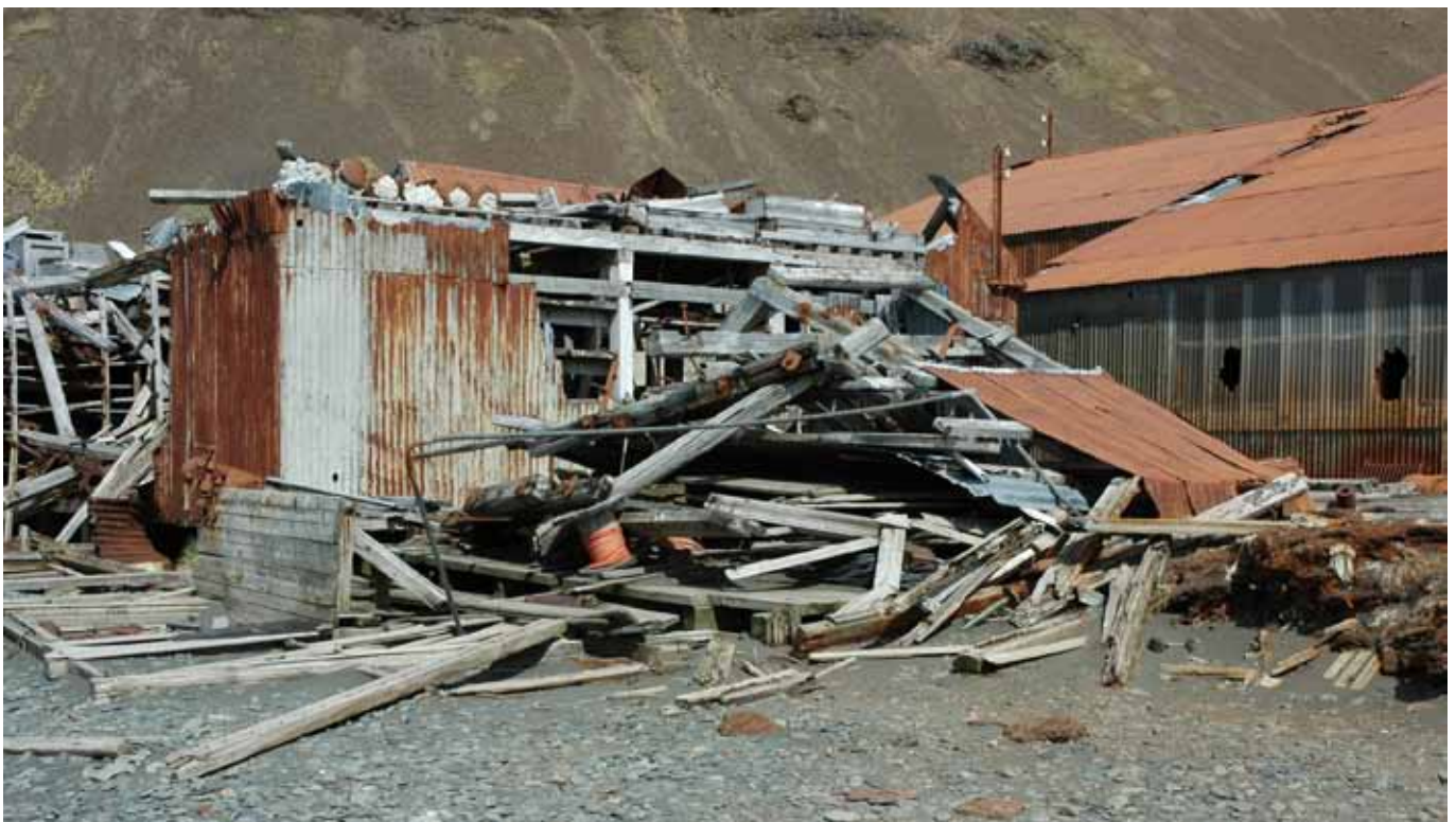
7.2 The east side of the collapsed building with Building No. 8 to the left and Building No. 6 to the right
