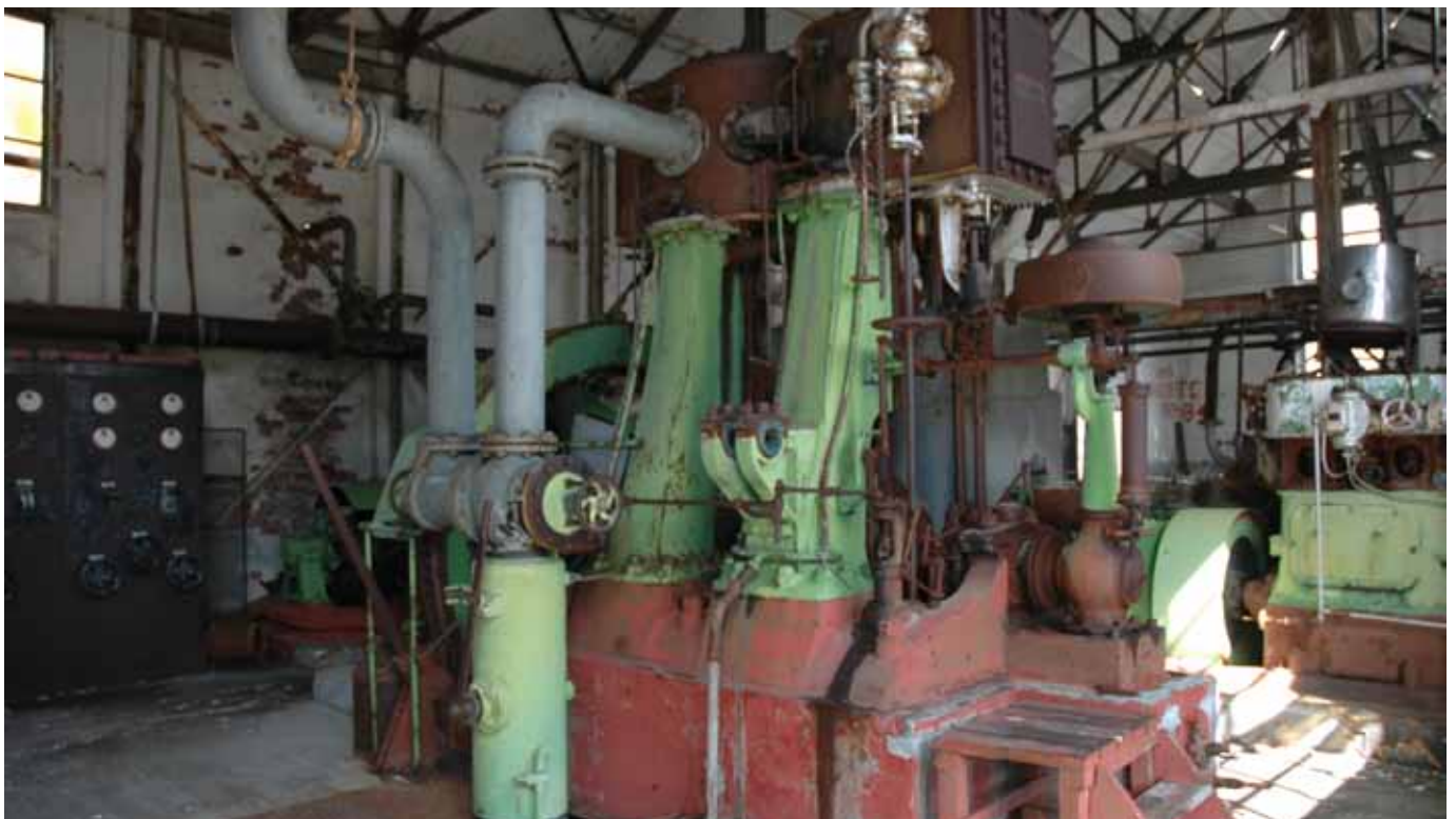
5.2.3 One of the two steam reciprocating dynamos originally made for the Bergen Tramway system
