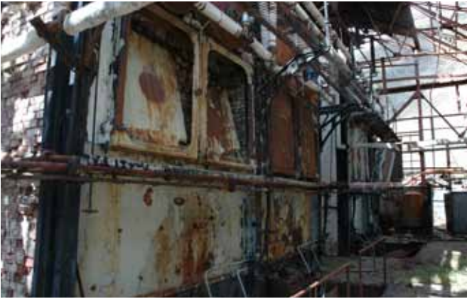
5.2.5 The main boilers
