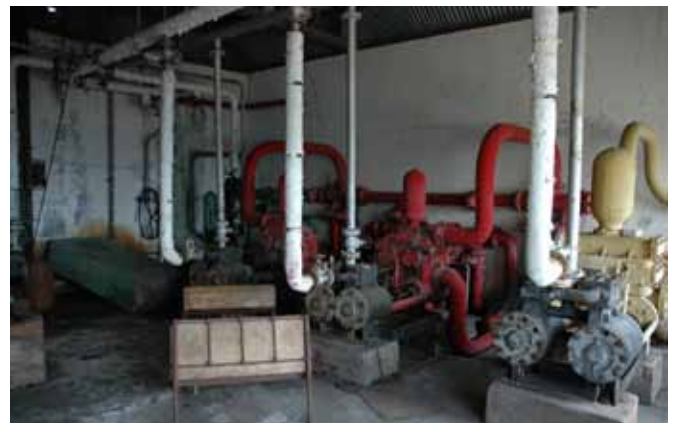
9.4 The remaining pumps
