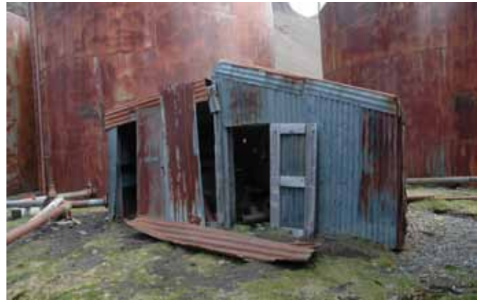
34.1 Pump House by Tank No. 48 (not on Bjorn Basberg's Plan)
