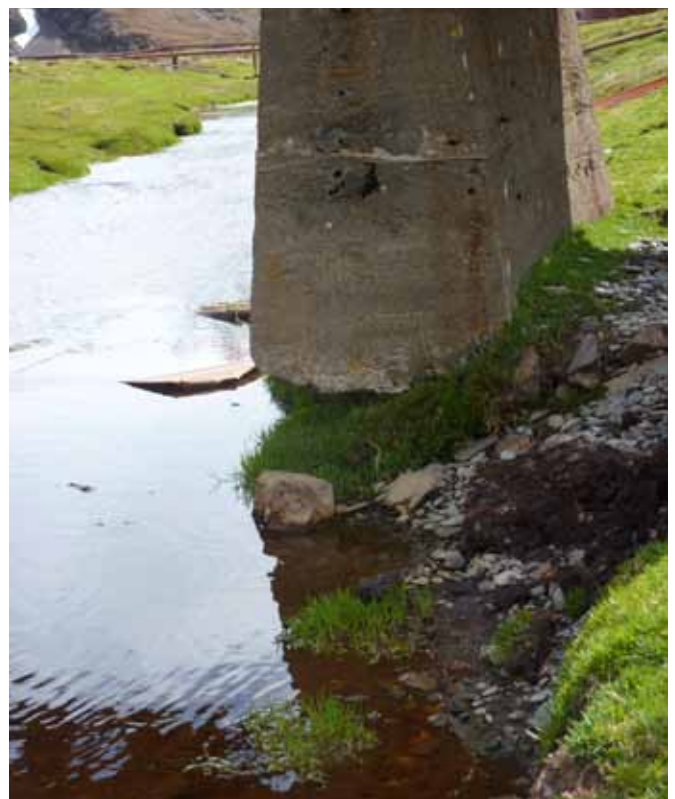
33.4 Concrete pier being undermined by the stream
