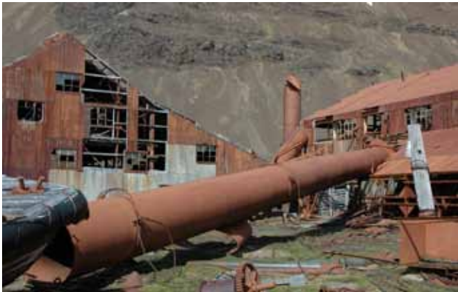
1.4 The fallen boiler chimney
