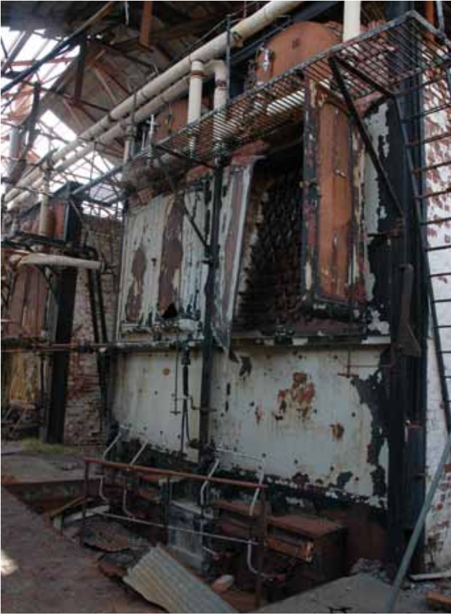
5.2.8 Detail of the Main Boiler
