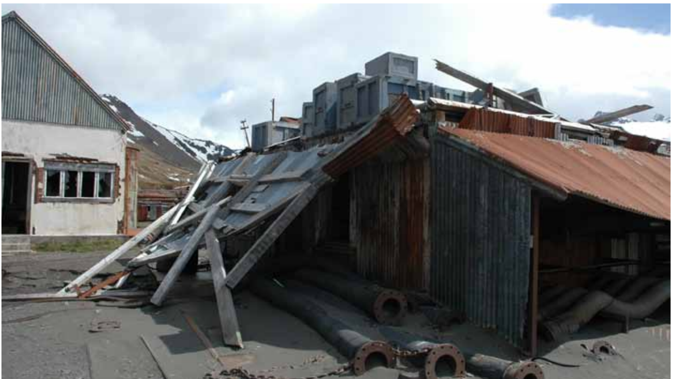
8.4 The south gable end with Building No. 9 in the background to the left
