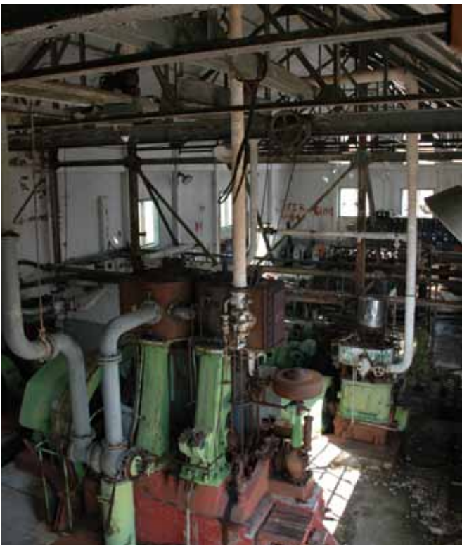
5.1.10 General view over the Power House looking west from the high level gallery
