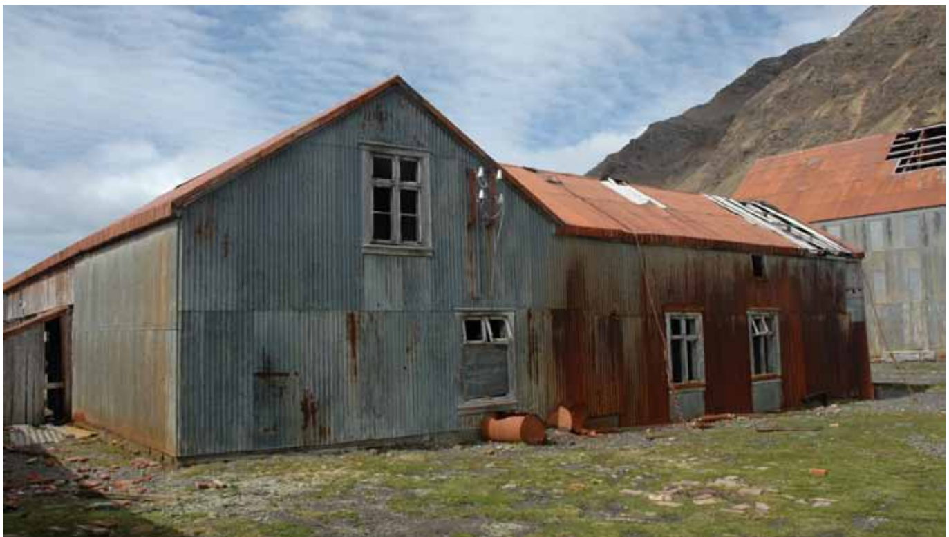
15.3 West elevation of the west wing and part of the north elevation and west gable of the north wing
