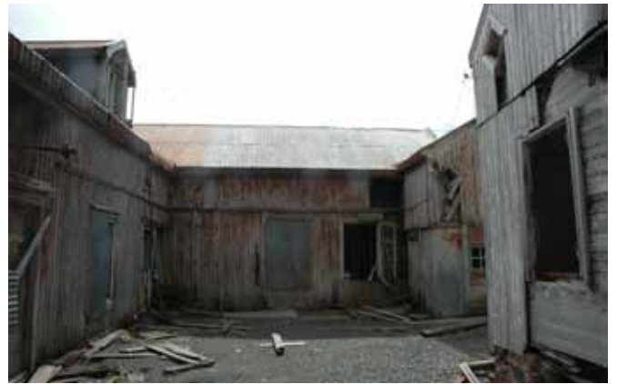
15.5 The south elevation of the north wing with the west wing to the left of the picture and Building No.16 to the right
