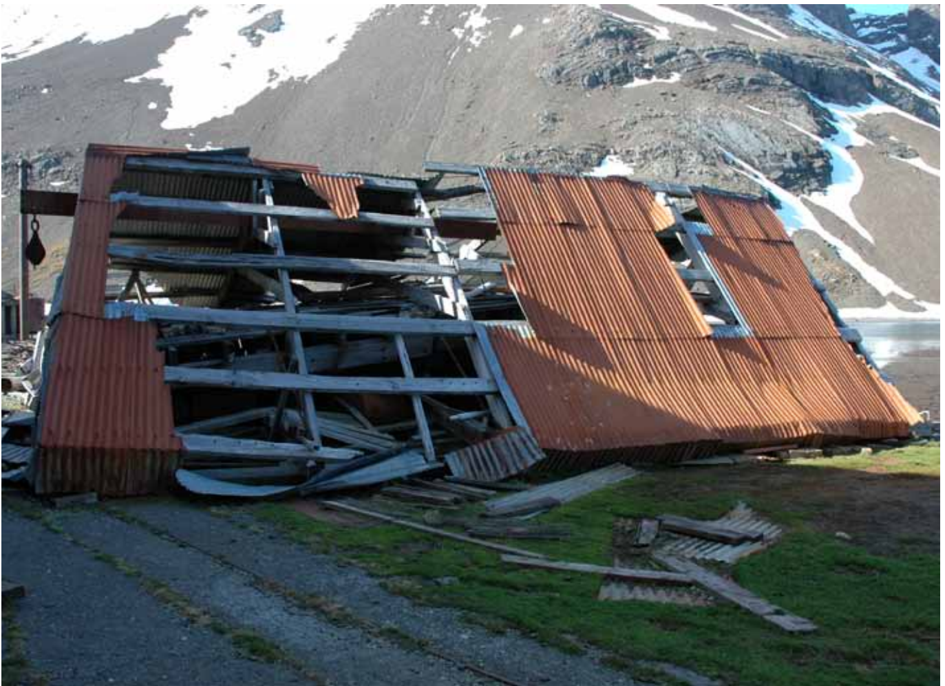
73.4 The south side of the roof which remains surprisingly intact
