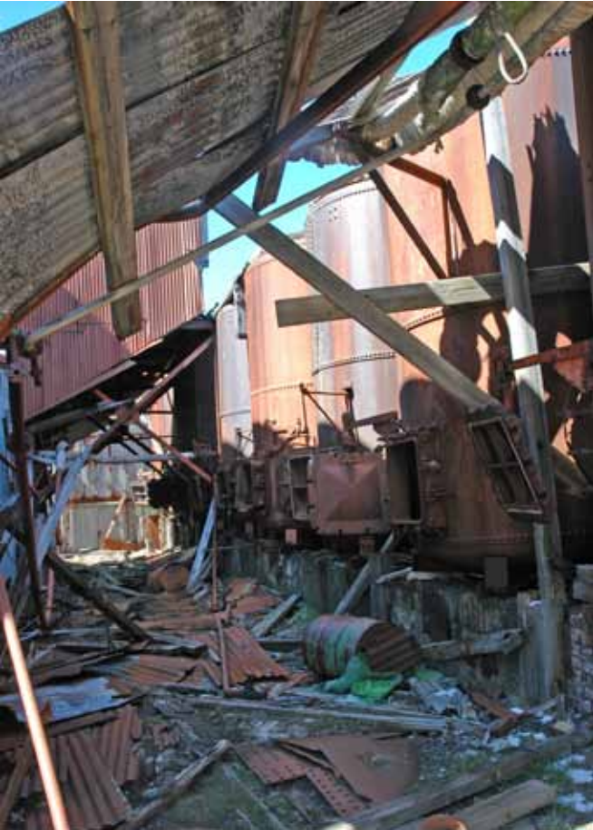
4.4 The north side of the building looking eastwards down the line of the cookers
