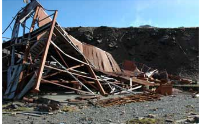
74.2 The northeast corner where the stanchions have ripped out of the concrete
