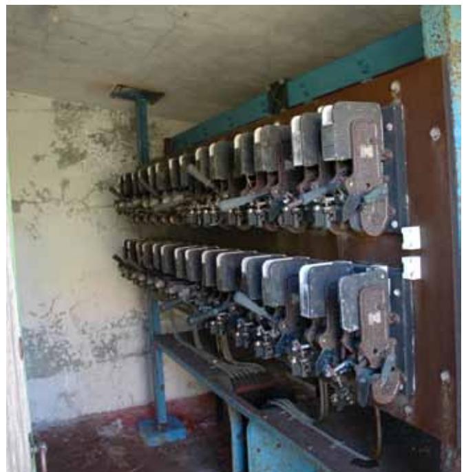
55.3 The remaining switchgear
