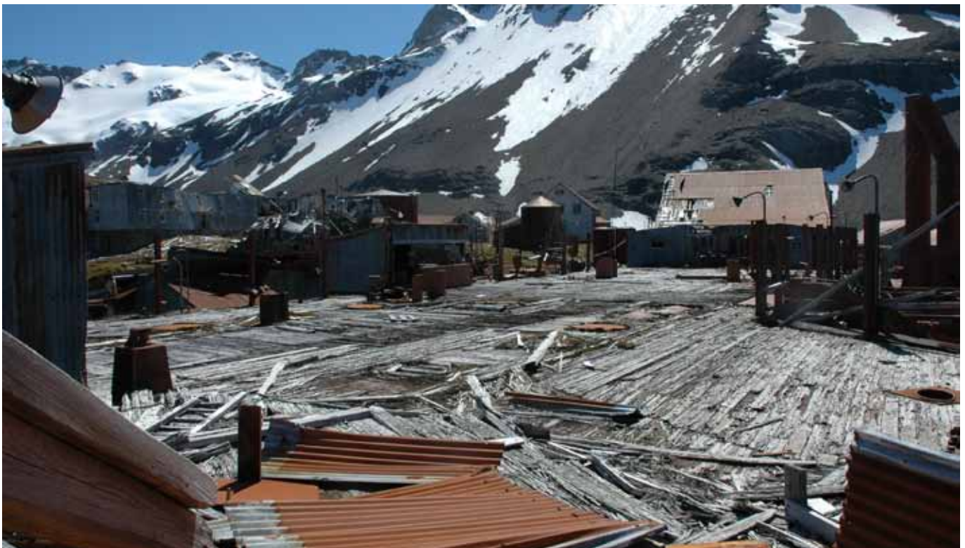
6.3 The loft over the Bone Cookery seen from the Rose Down building
