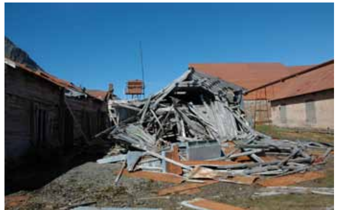
53.7 The collapsed northwest end of the main (northwest-southeast) wing
