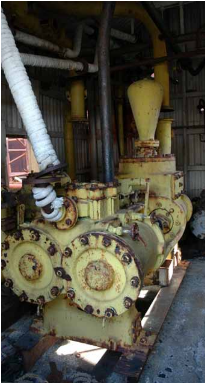
69.2 Detail of one of the pumps
