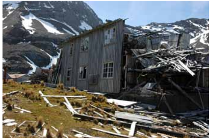
44.2 The remaining section of wall on the west side of the building
