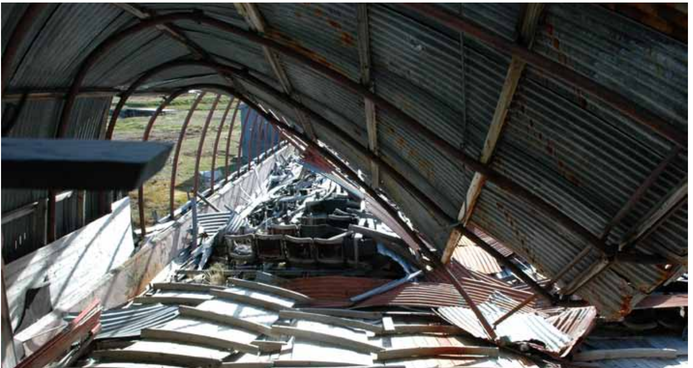
80.6 Looking west under the collapsed roof from the east end
