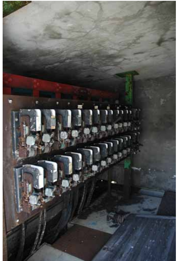
41.2 The remaining switchgear
