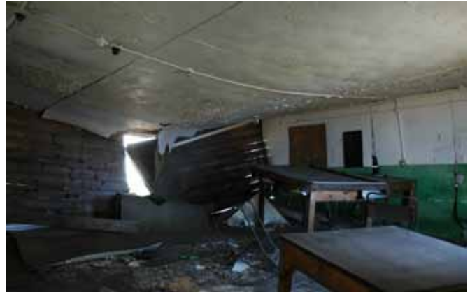
46.3 The interior of the main space showing the collapsing roof
