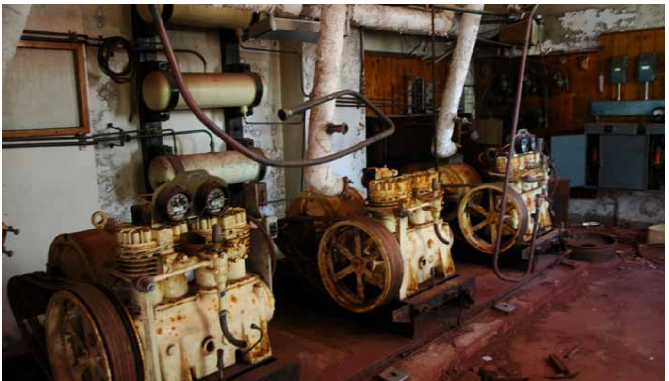
35.5 The mechanical plant in the northern ground floor room
