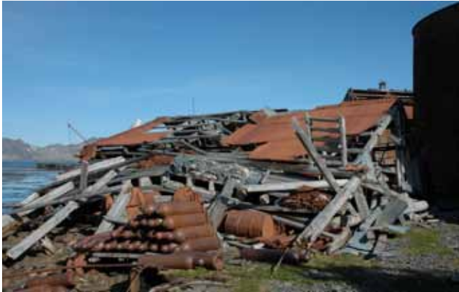
73.1 The collapsed building seen from the north
