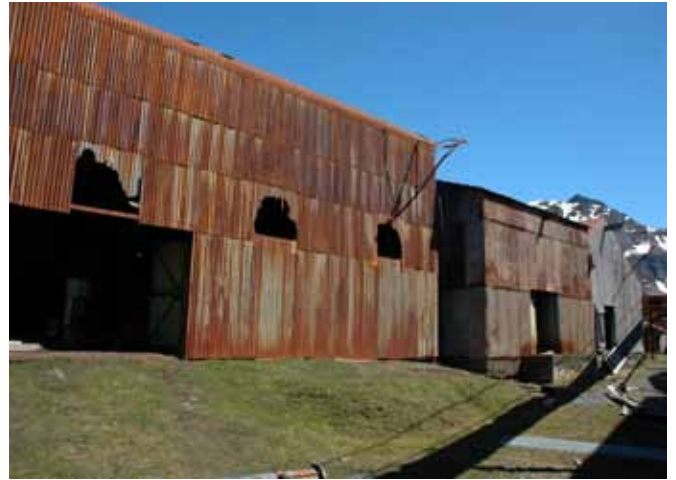
10.4 The west end of the north elevation showing the two big outshots
