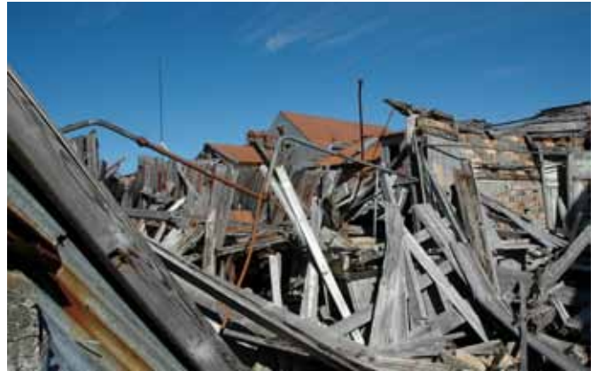
63.1 The central section where the fittings remain under the collapsed roof
