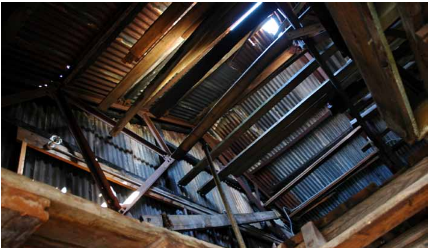
32.6 The roof structure seen through the access hatch to the storage loft
