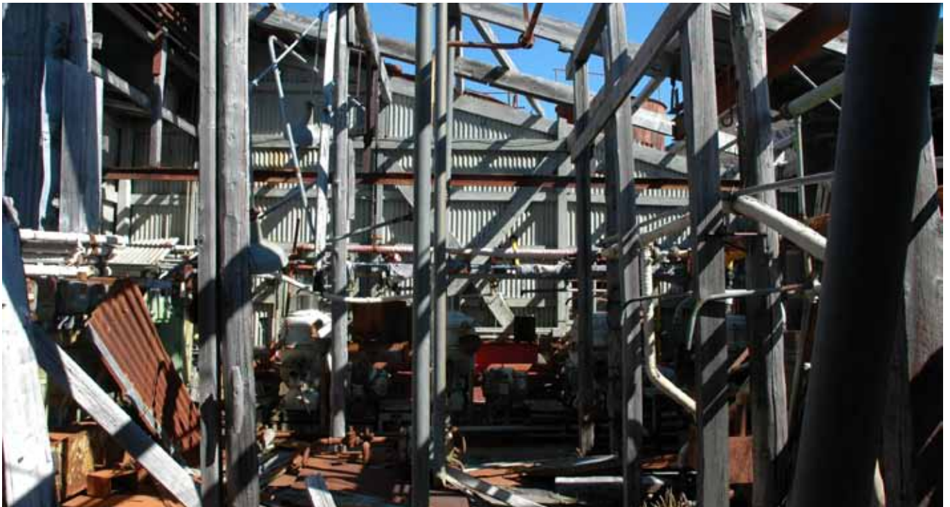
22.3 The collapsed central area
