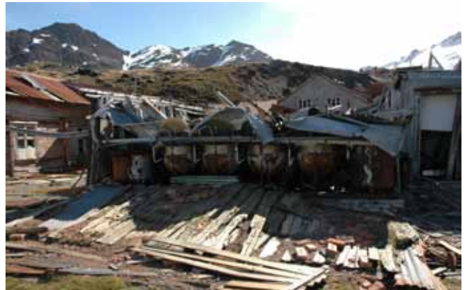
63.4 The east end of the buiding which has collapsed completely
