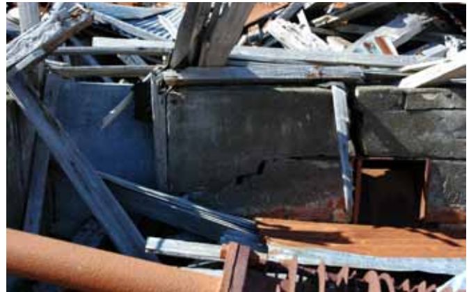
33.1 The pig pens inside the collapsed building
