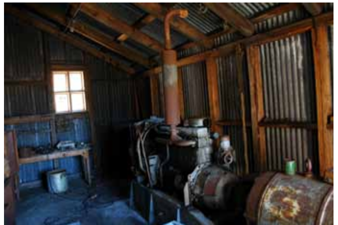
36.5 Generator in the northwest lean-to
