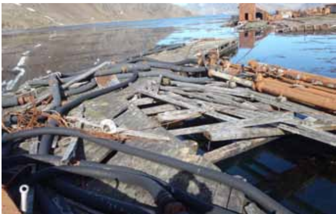
87.3 Looking along the Pier southwards with the Quay and Coal Store (No. 62) in the background
