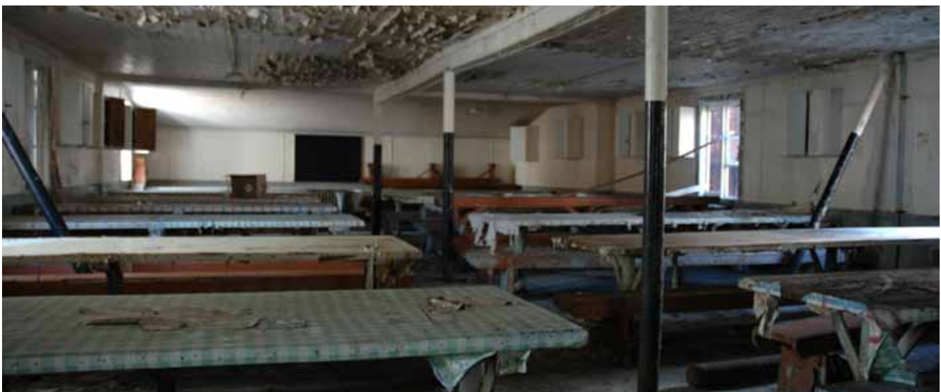
63.6 The interior of the Main Mess in the west end of the building
