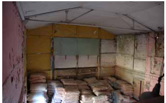
19.2 The interior of the store (Old Cinema) looking west with the old screen still invisible on the end wall
