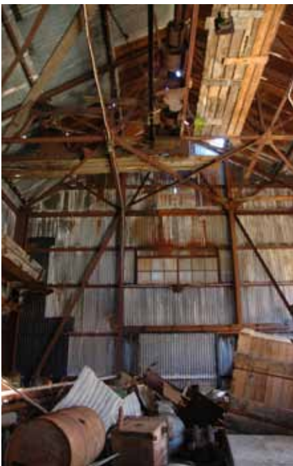
10.5 The interior of the west end of the two northern side outshot buildings
