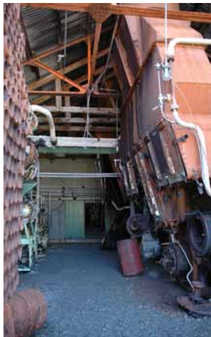
10.6 The boilers in the Boiler House in the South West Wing
