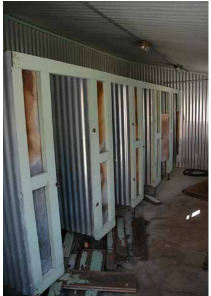
15.2 The interior of the WC Block (the northern part of the building)
