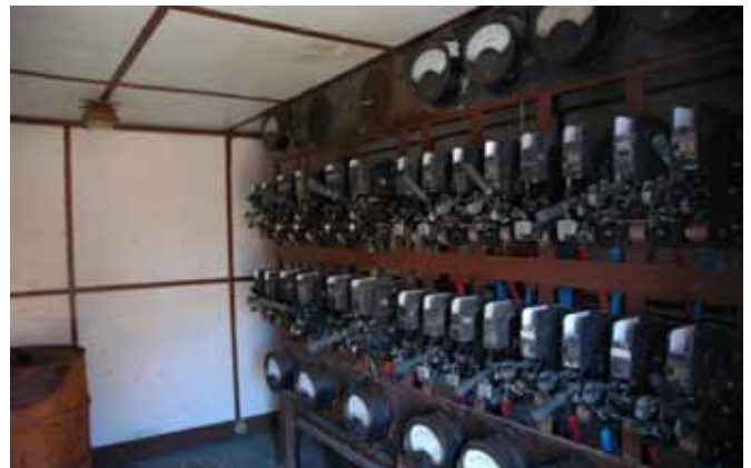
20.2 The electrical switch room
