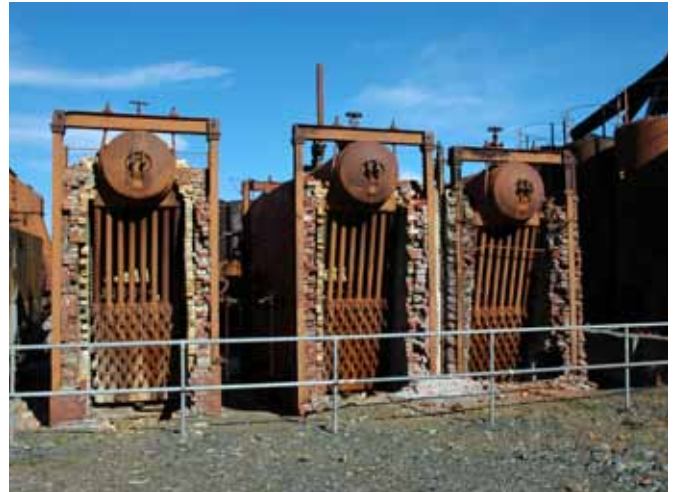
3.6 West end of boilers
