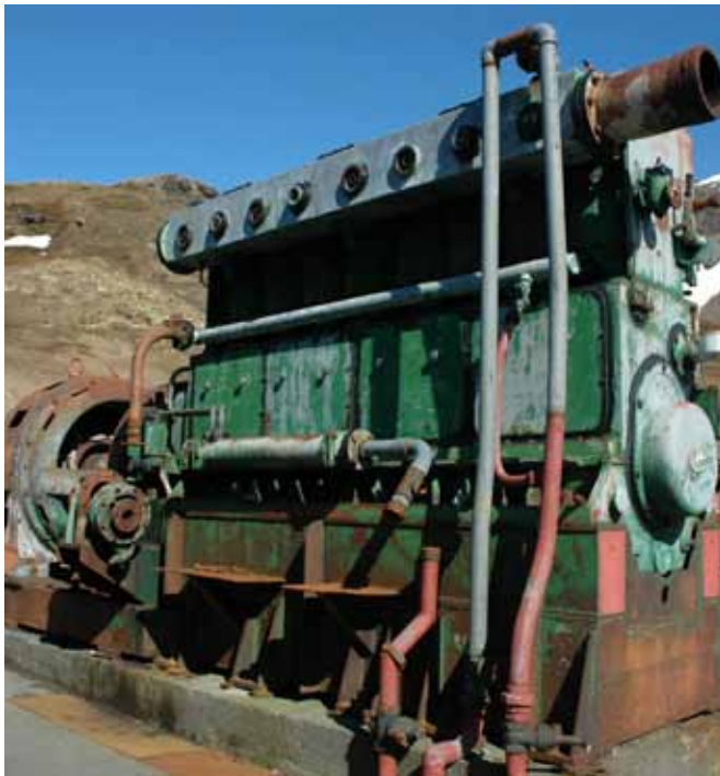
23.3 Diesel electric generator set
