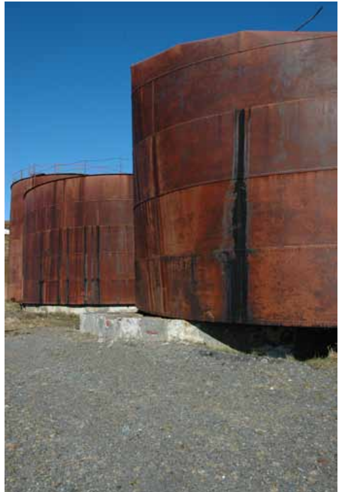
78.1 Tank displaced off its base by the salvage work
