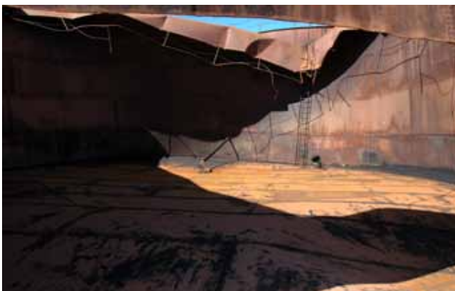
78.2 The typical way a Tank collapses once the roof falls in
