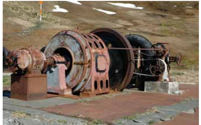
23.1 Hydro electric set with covering still in place on the generator
