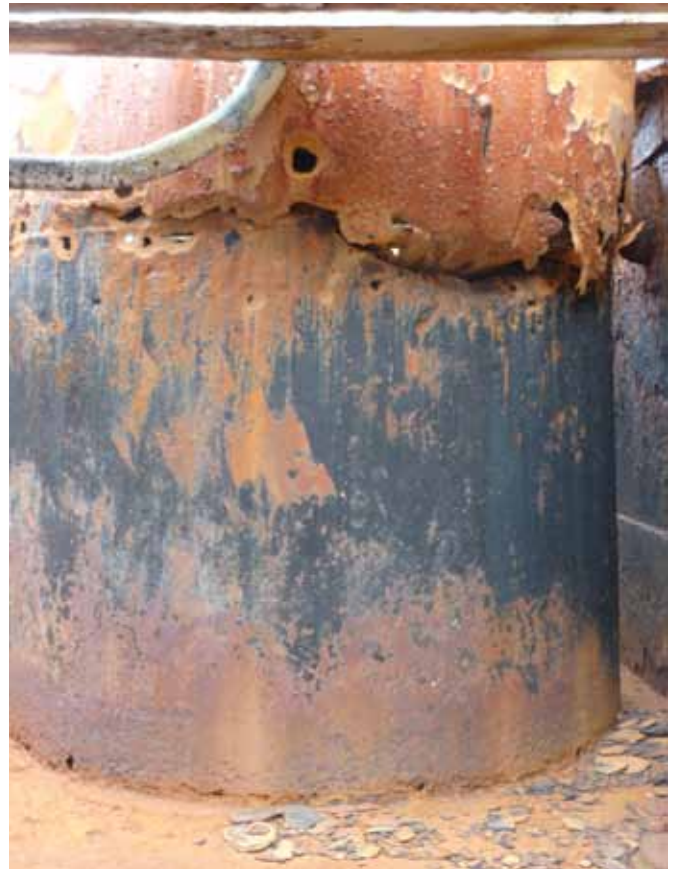
52.5 The corrosion allowing the funnel to collapse and tip over
