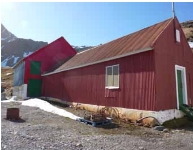
46.2 The Slop Chest entrance in the east elevation. The later taller extension can be seen in the background.
