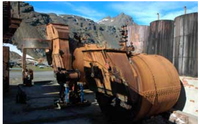
3.7 Second row of boilers looking northwards
