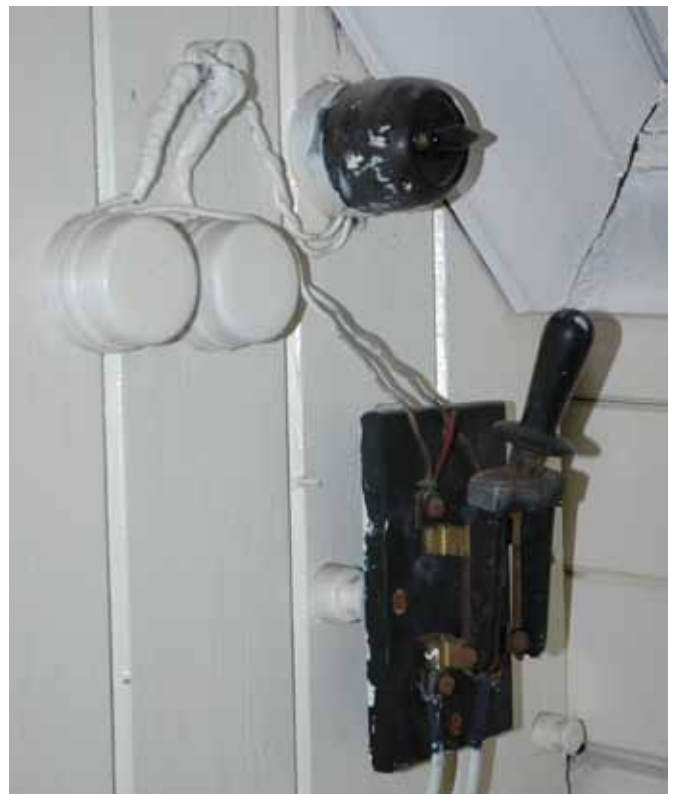
34.11 Remnants of the old electrical system (now disconnected)
