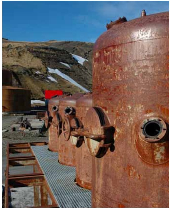
5.2 Detail of boilers
