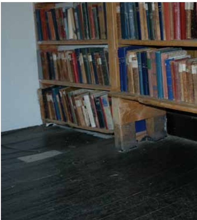
34.14 Bookshelves on the east wall tipping where the floor is sinking
