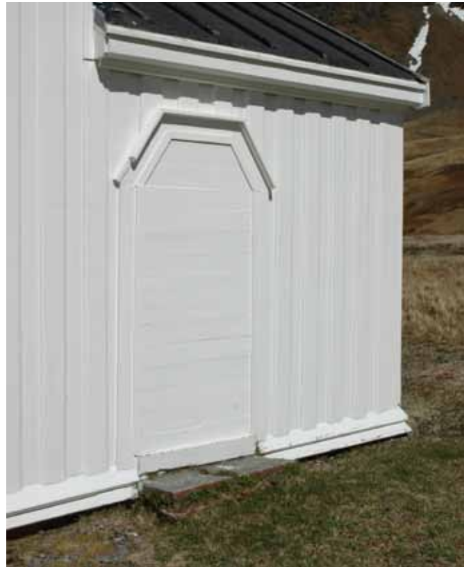
34.8 The blocked north door
