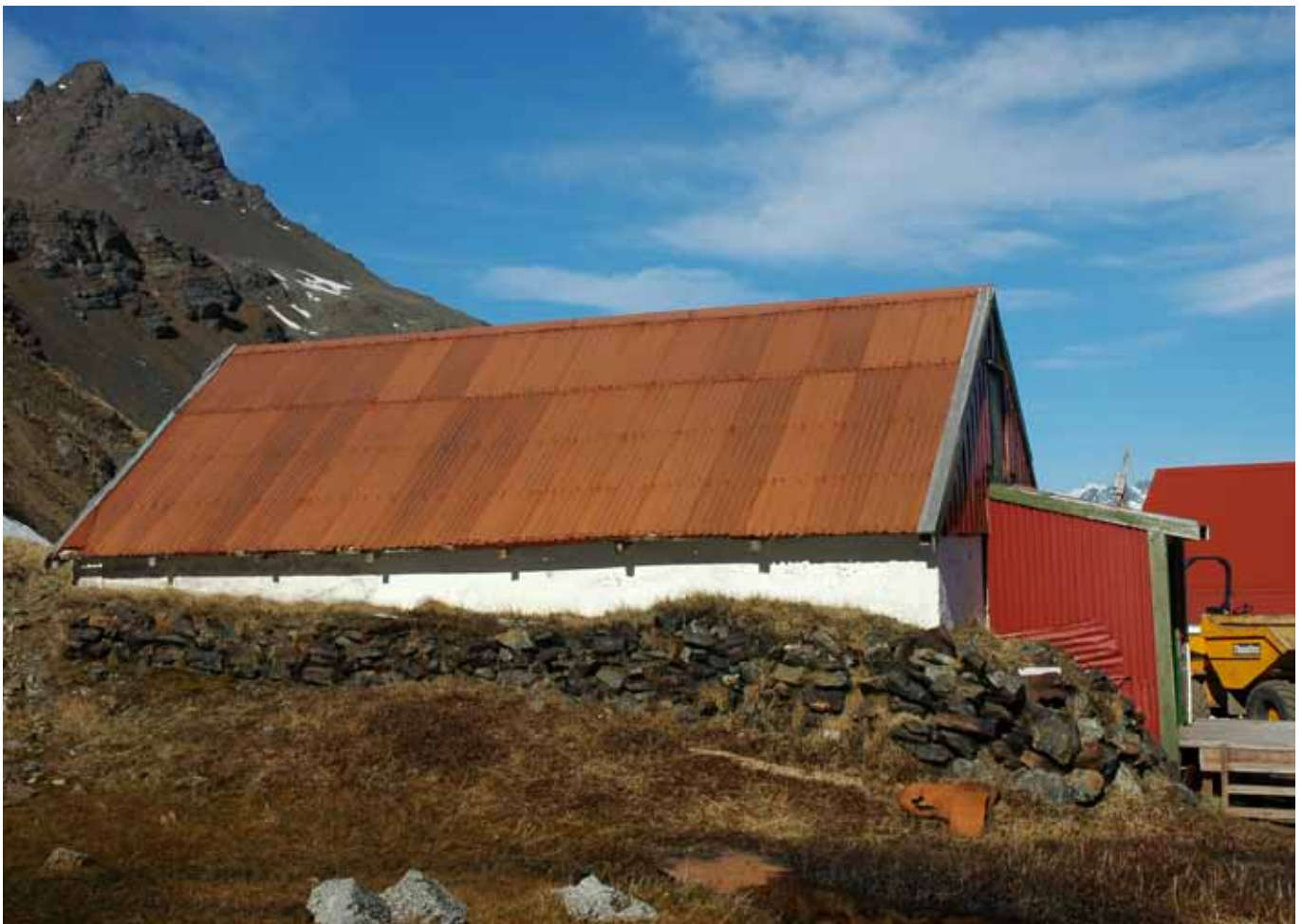
41.2 The west elevation with rock piled up against the walls
