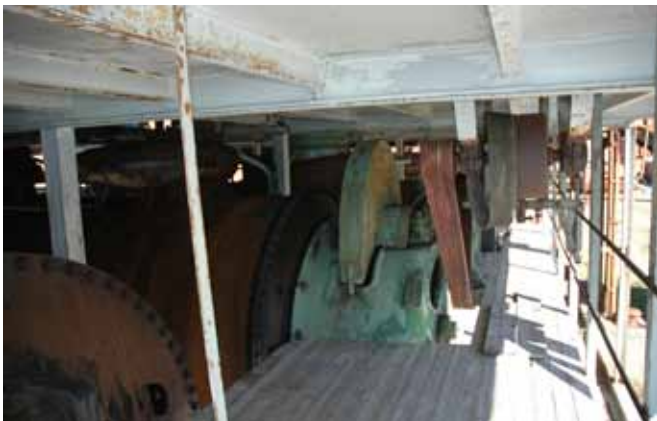
2.16 Floor immediately under the open deck of the Meat Cookery with ovens still in place
