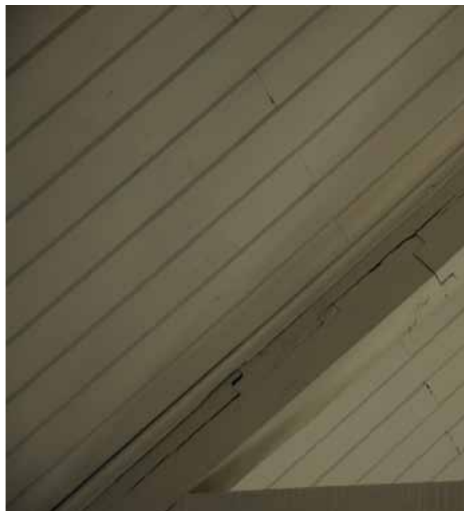
34.15 Cracking in the principal beams
