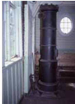
The gap behind the brick wall shows how the building leans.
