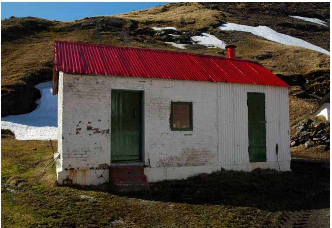
45.3 The southeast elevation; the later extension to the northeast can be clearly seen
