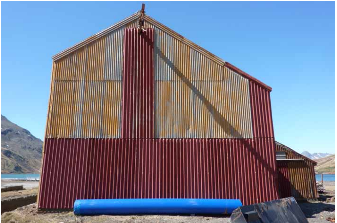
10.4 West elevation showing the extent of the repair in modern sheeting of the wrong profile
