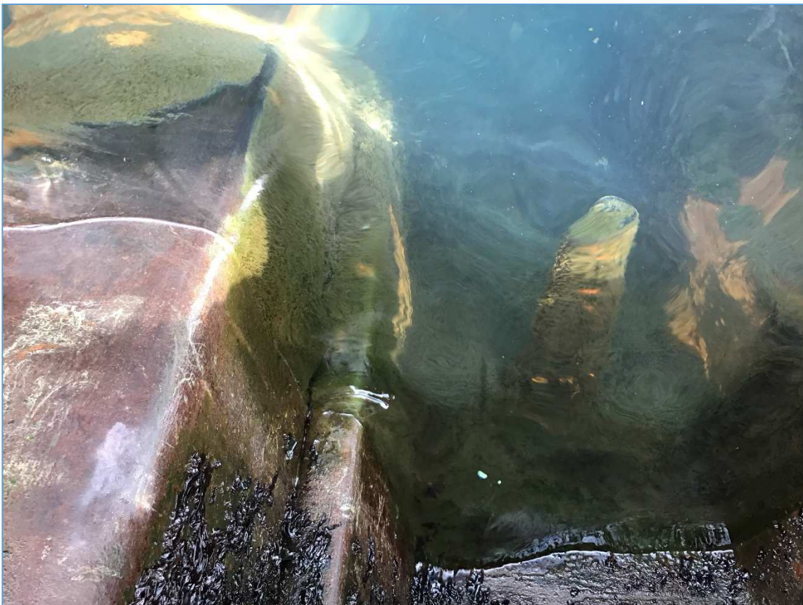
Top view on sheet piles and tie rod on south wall – note threads on tie rod visible
