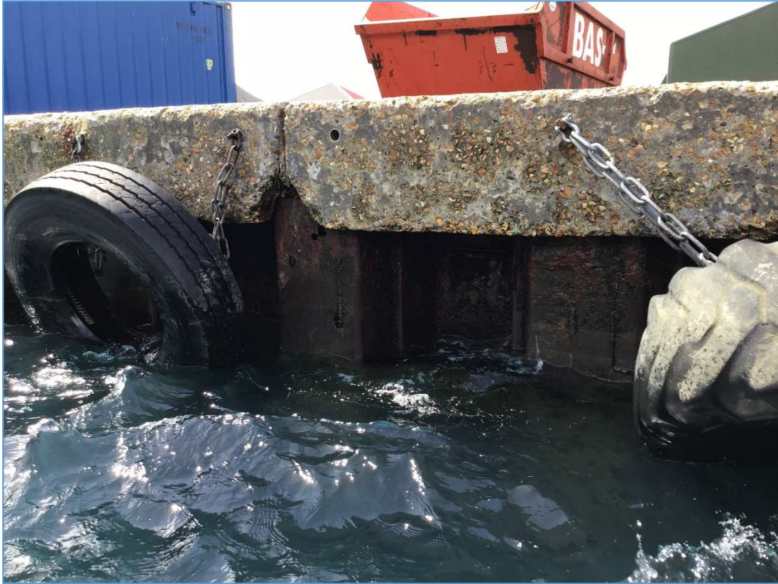
Capping beam – exposed aggregate on front face and missing corners at ends of beams
