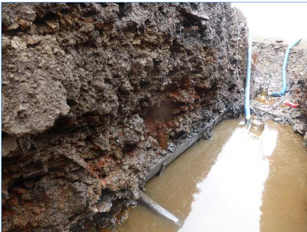
Waling beam to anchor wall and connecting inclined tie rod to front wall
