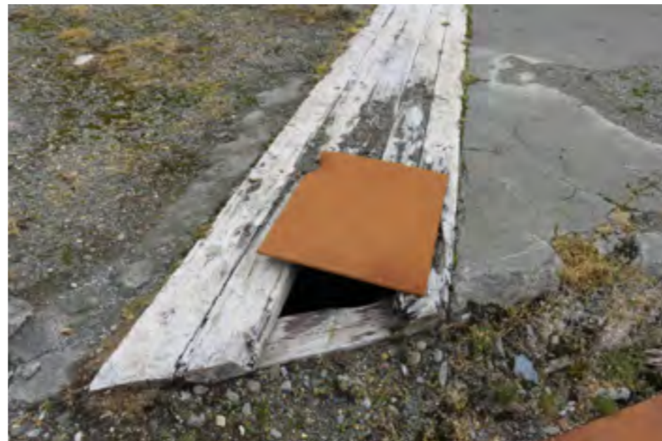
Hole over the culvert in the Guano Store
