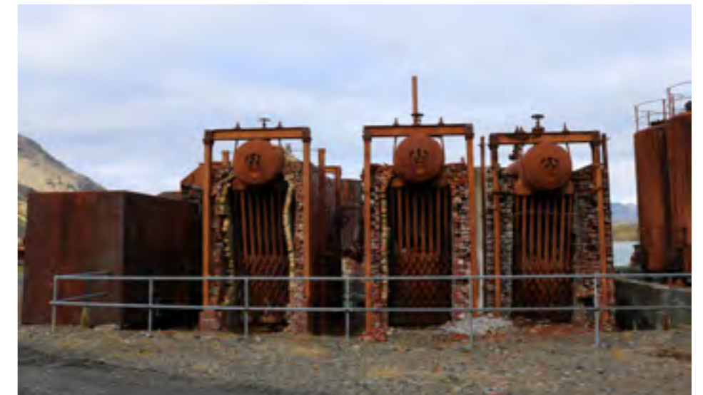
Barrier in front of the boilers with failing brickwork in the Boiler House
