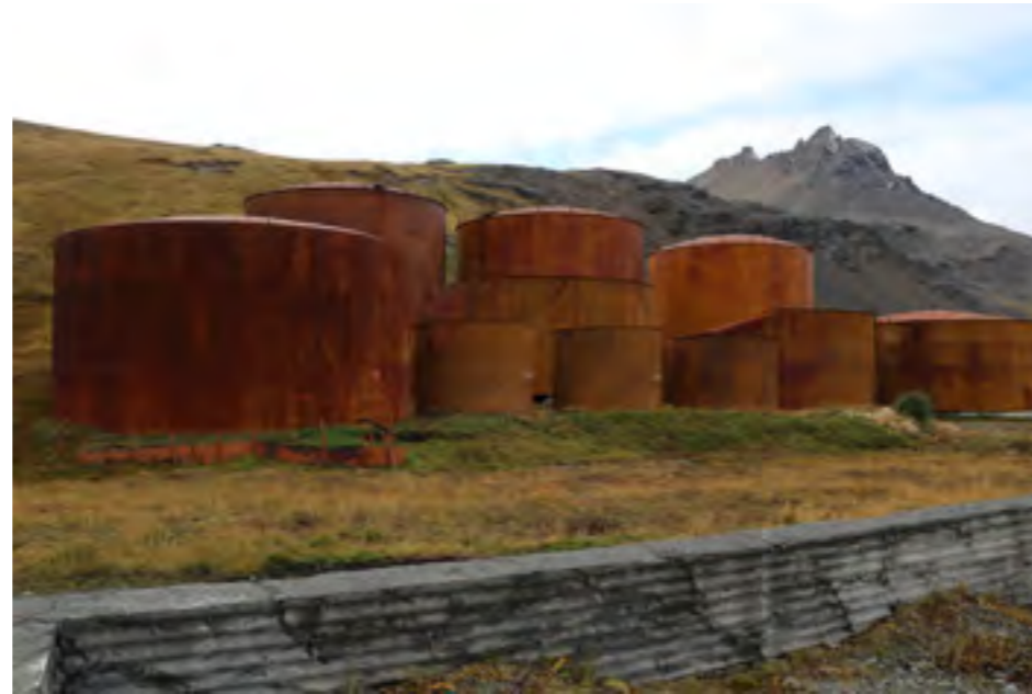
North-west storage tanks
