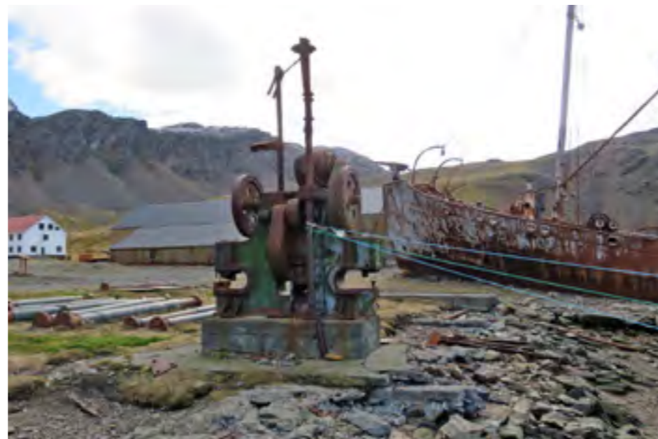
The Plating Store floor is crumbling due to the effect of the sea
