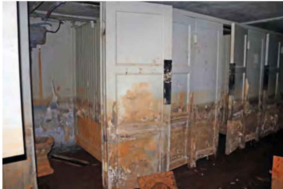
Evidence of past flooding in the Nybrakka basement
