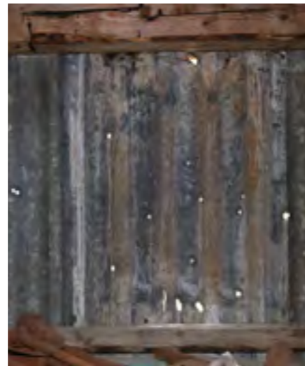
Bullet holes in the Main Store wall
