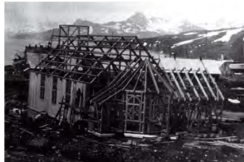
Construction of the frame of the Church in November 1913, reproduced courtesy of the South Georgia Museum
