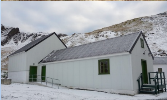
The Slop Chest during re-roofing (above) and following the completion of the external work (below).
